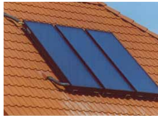
Solar collector device on the roof of a single-family home
