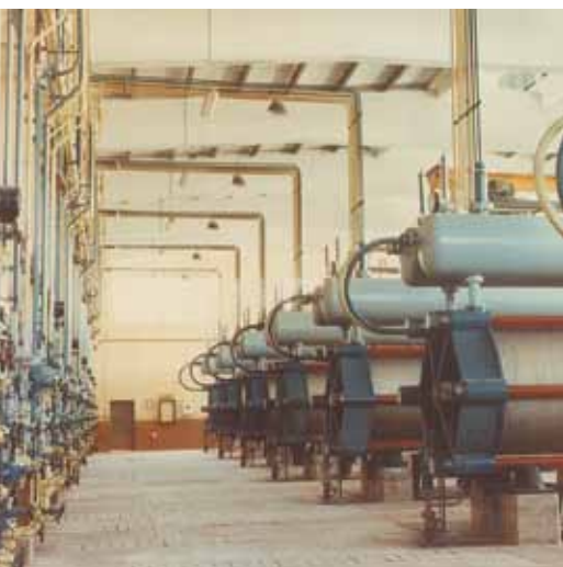
Industrial hydrogen production by the Lurgi pressure electrolysis process (Lurgi factory photo, Germany)
